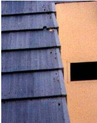
Possible roosting/nesting attempts along with drumming damage on cedar shakes
