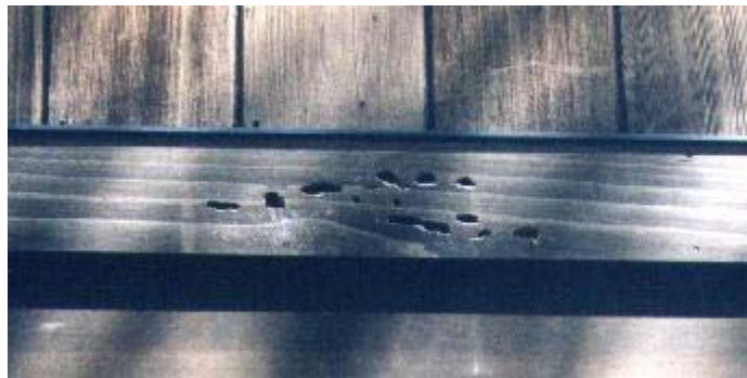
Figure 11. Woodpecker damage due to foraging for carpenter bee larva on cedar trim boards of a house
