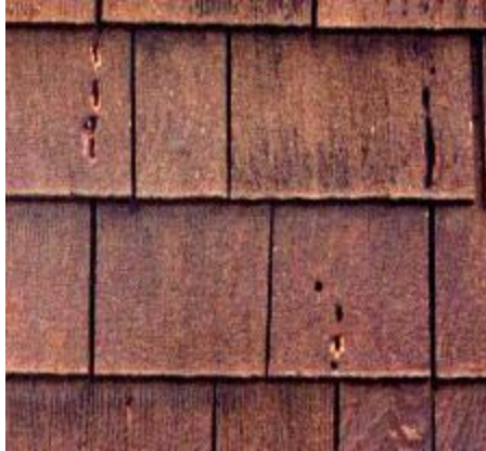
Figure 5. Damage due to woodpecker foraging for insects on cedar shingles
