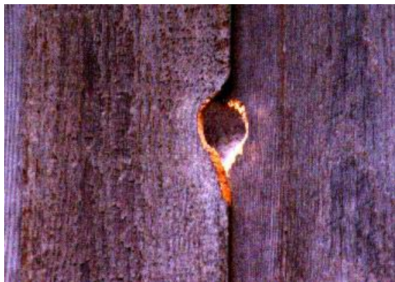
Figure 8. Nesting/Roosting cavity on stained cedar board-and-batten
